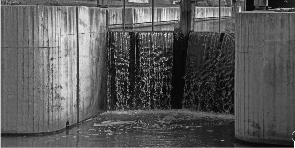
Figure 32: Photo of the east end spillway looking upstream at the retaining wall for the lake. Notice the size of the dry laid dressed limestone blocks. Source: https://seemore.org/play/lake-life/the-aqua-life-at-grand-lake/
